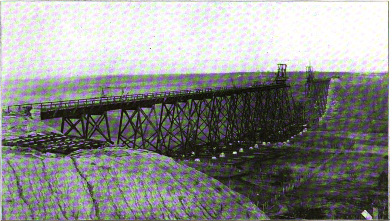
VIADUCT AT BOONE, IOWA, CHICAGO & NORTHWESTERN RAILWAY—SHOWING TRAVELERS AND FALSE WORK IN PLACE PREPARATORY TO ERECTING CHANNEL SPAN. From photograph taken March 18, 1901.
